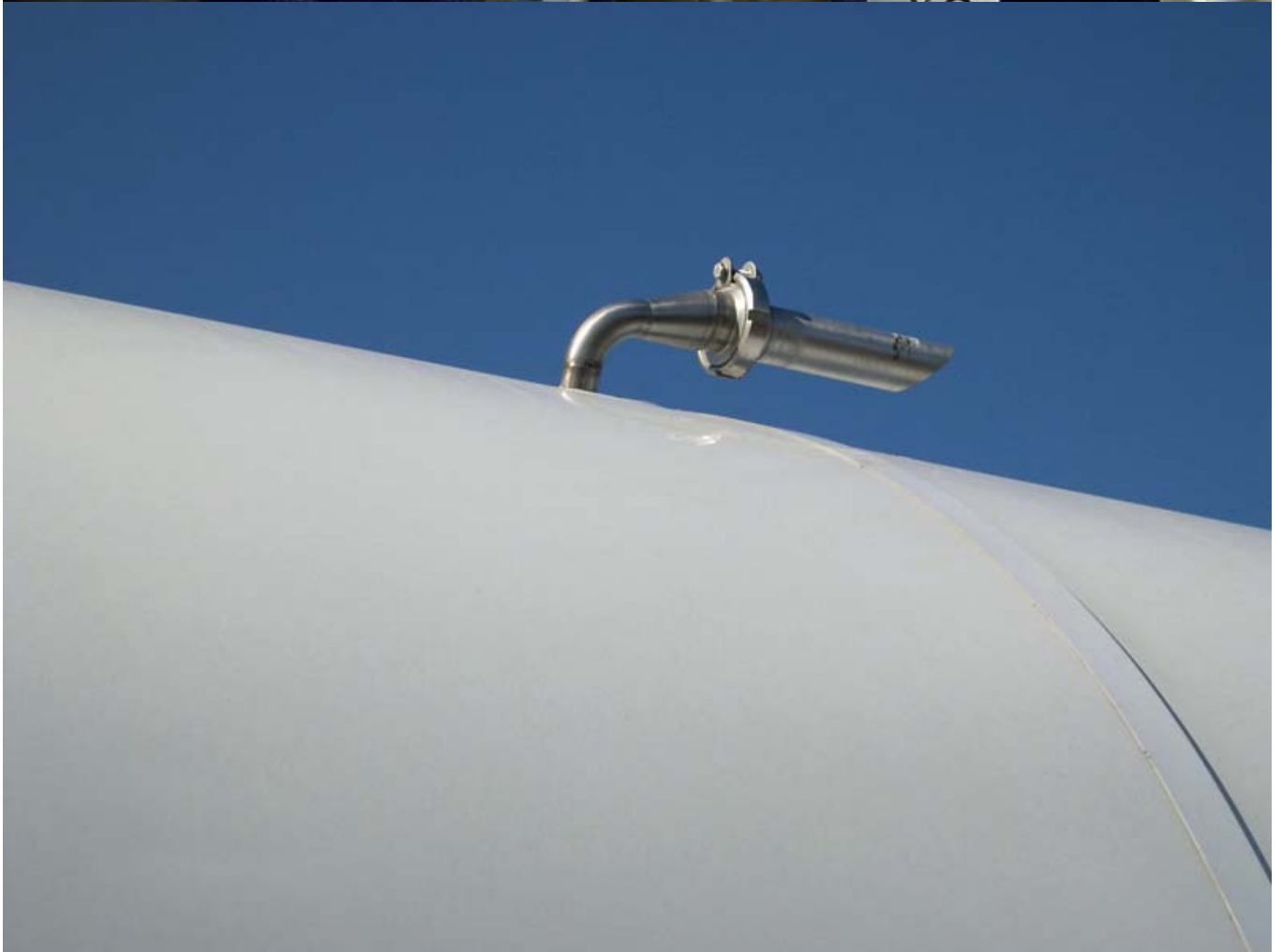
Figure 8. Safety valves and venting device. Source(4): Authors.
