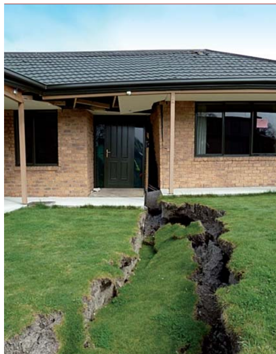
Figure 10: Example of a total loss of a residence in the eastern suburbs due to lateral spreading (left). (Photo: Tonkin & Taylor Ltd).
