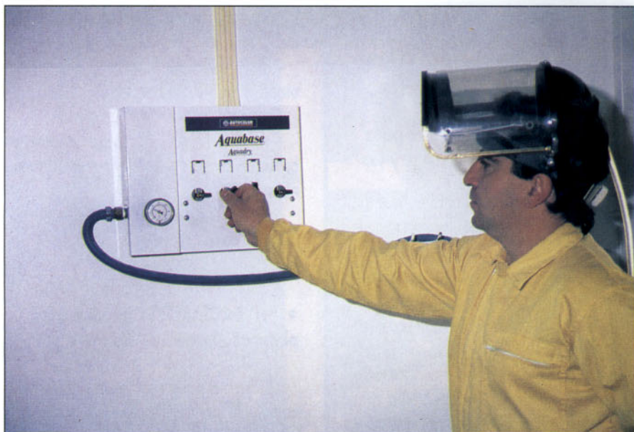
Panel de control.
