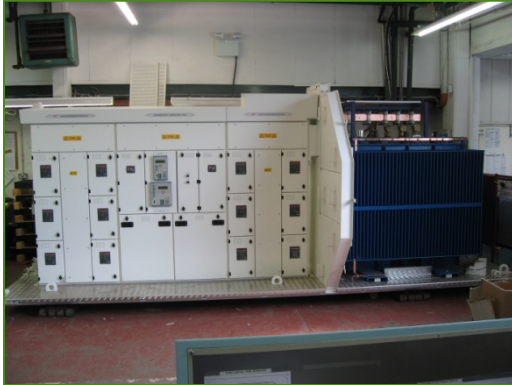
USP Electrical Internals
