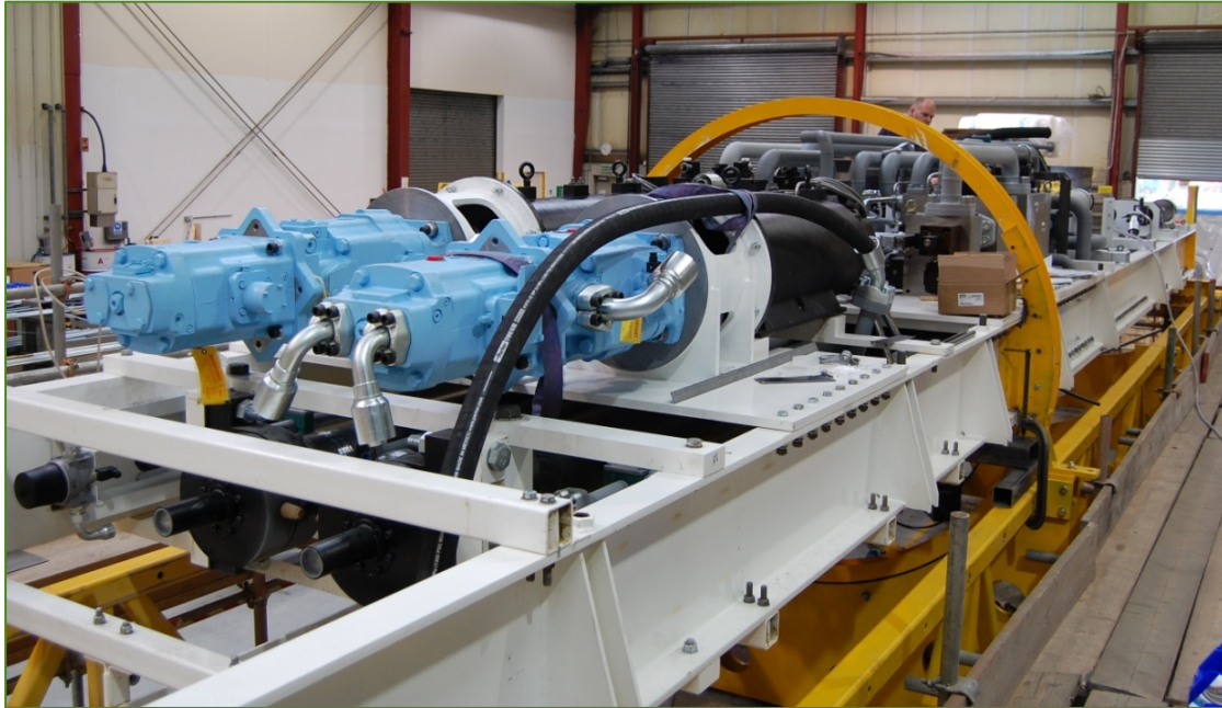
PB150 Power Take-Off System, Warwick, UK
