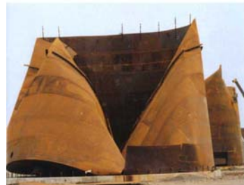
Fig. 15: Tank farm after windstorm [© MR]
