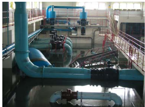
Fig. 12: Power plant after Flood
